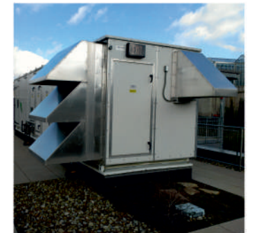
• Energy Recovery System
