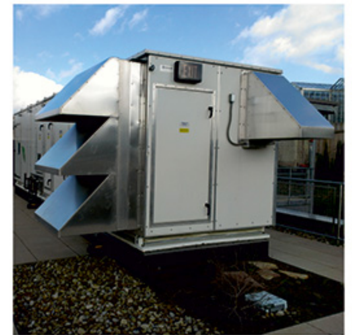
• Energy Recovery System
